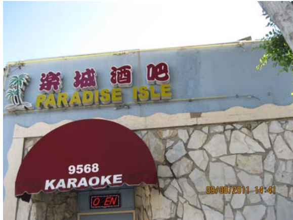
(Before) Peeling/chipping paint and non-operable lighting.
