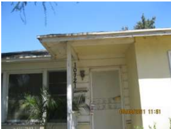
(Before) Weathered siding, chipping/peeling paint and dilapidated fence.
