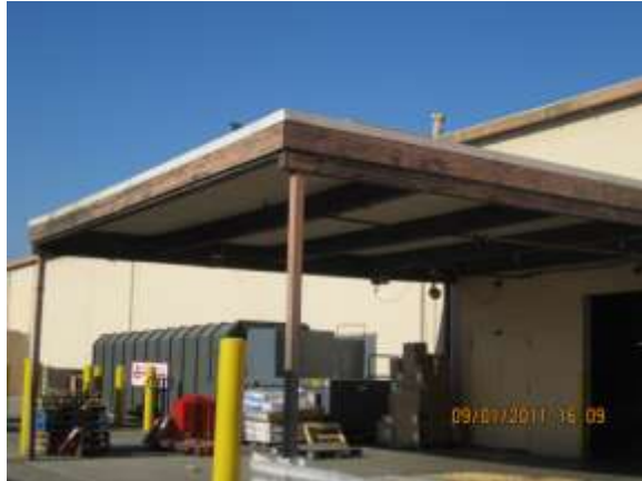
(Before) Peeling/chipping paint on patio cover
